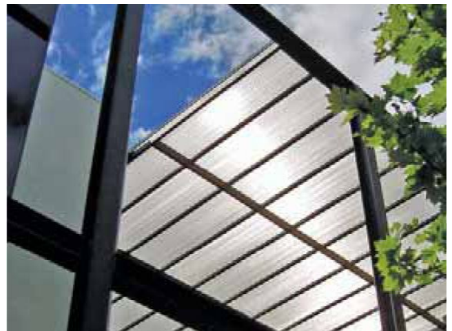
Devices that enhance a building’s energy efficiency can also provide a strong architectural identity
