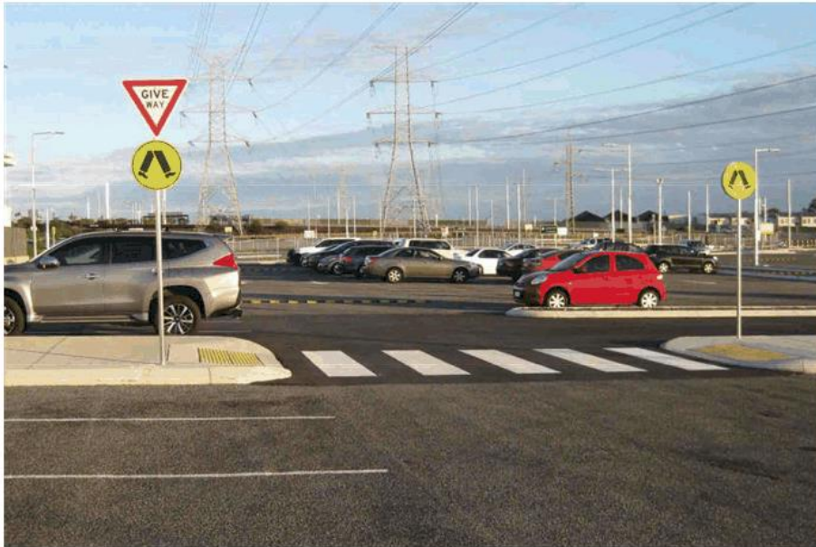
Photo 5: Give Way sign incorrectly installed at a zebra crossing in the northern car park
