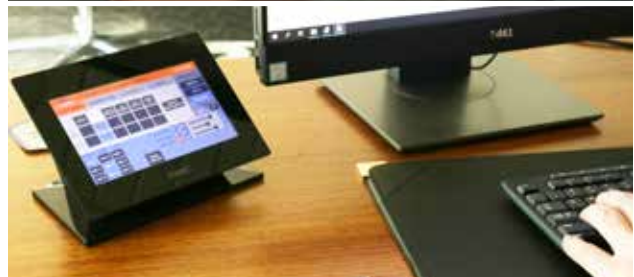
Nick from IT works on the Council Chambers audio visual equipment upgrade
