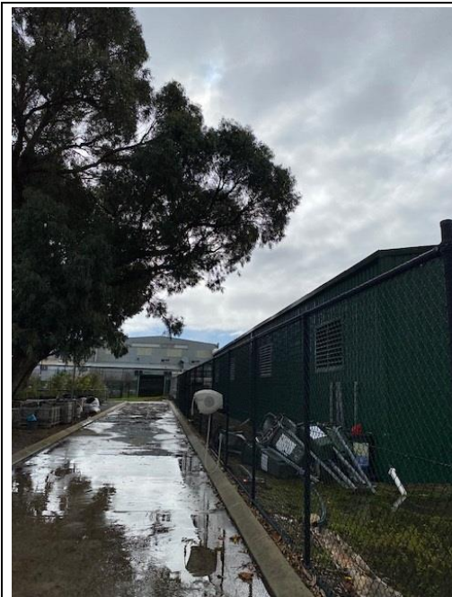
Image 5: Trees overhanging infrastructure
