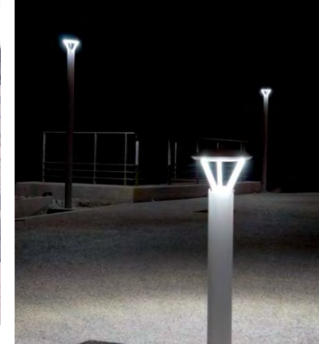
Bollard and overhead lighting
